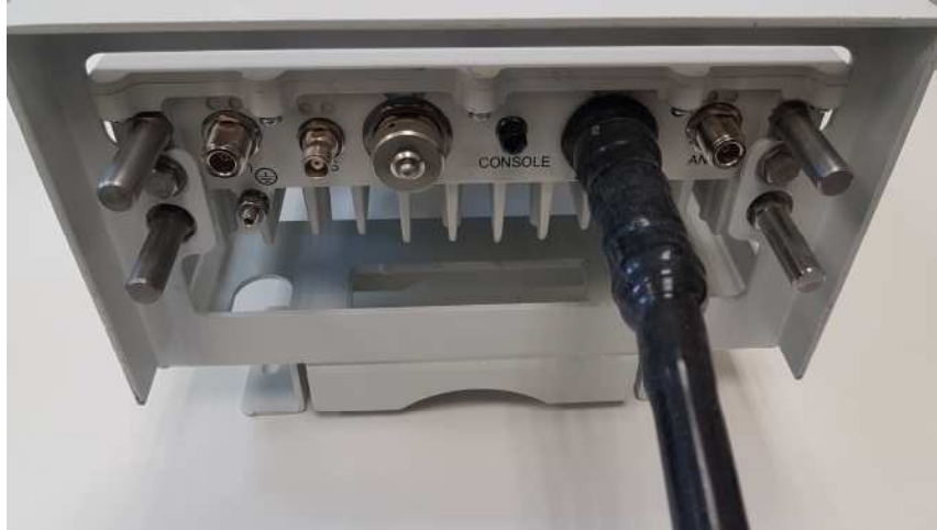
Figure 2-1: Cable Weatherproofed with Cold Shrink Tubing
