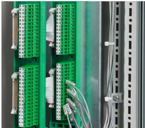
Figure 10-89 Terminal Module Cabinet
