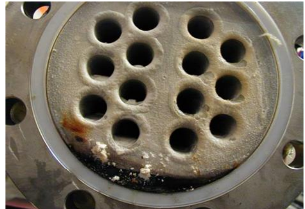
Figure 4-2: Fouling of tube bundle heat exchanger
