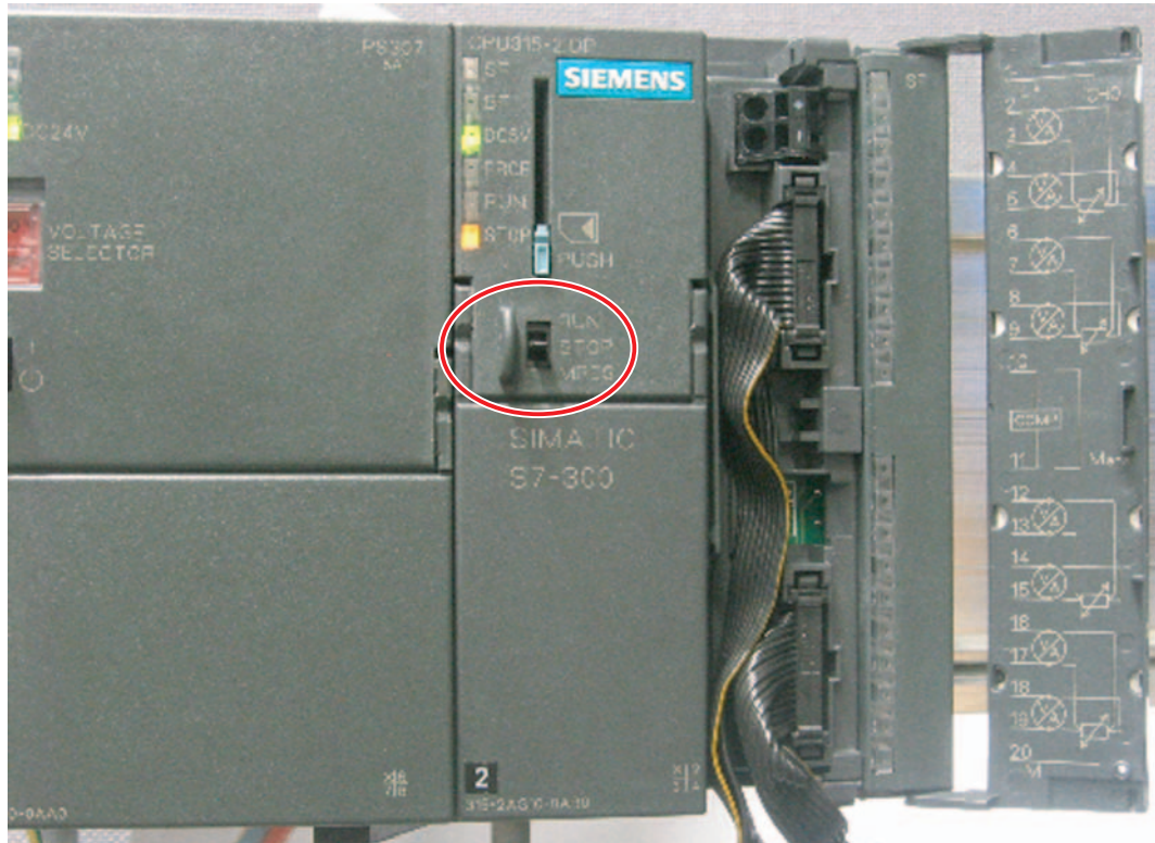
Figure 5-11 Successful wiring, CPU in STOP position
