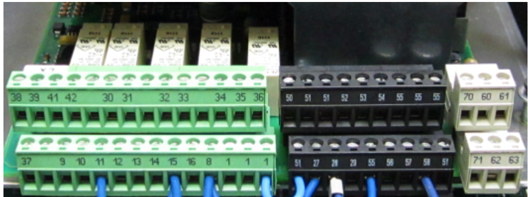
Figure 8-13 Control cable terminals
